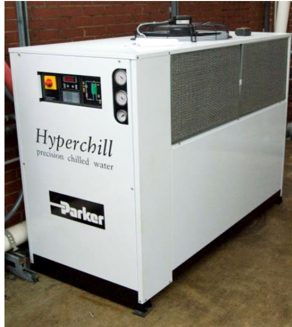
Figure 27 Hyperchill water chiller for air stream conditioning on FI test stand
