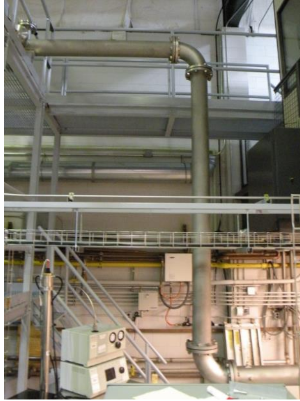
Figure 16 FI test stand downstream piping elevated section
