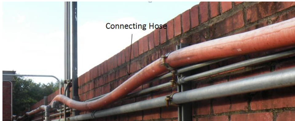
Figure 22 FI test stand rubber hose connecting claw compressor to air tanks
