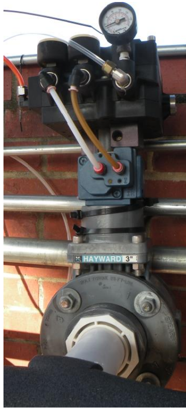
Figure 25 Pneumatic bleed off valve for FI test stand
