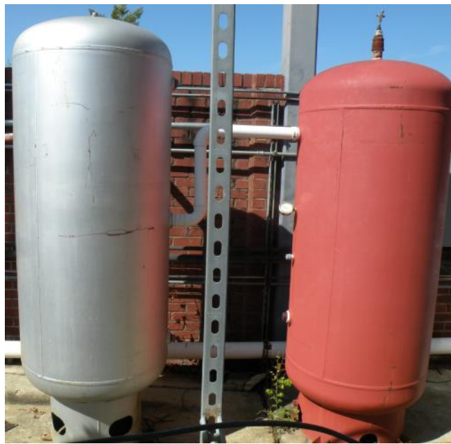
Figure 23 FI test stand buffer air tanks
