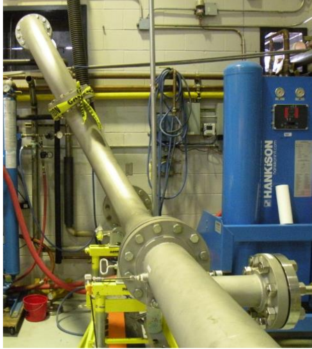
Figure 15 FI test stand upstream piping entering building
