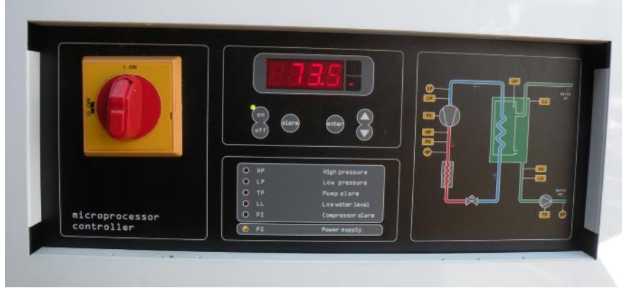
Figure 30 FI test stand chiller control panel
