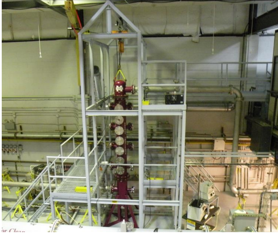
Figure 13 FI test stand and support structure
