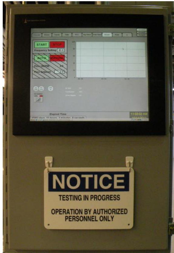
Figure 32 FI test stand control system computer with touch screen display
