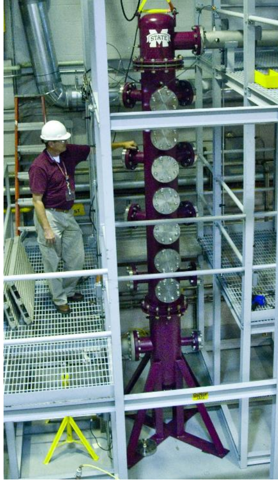
Figure 17 Assembled FI test stand housing
