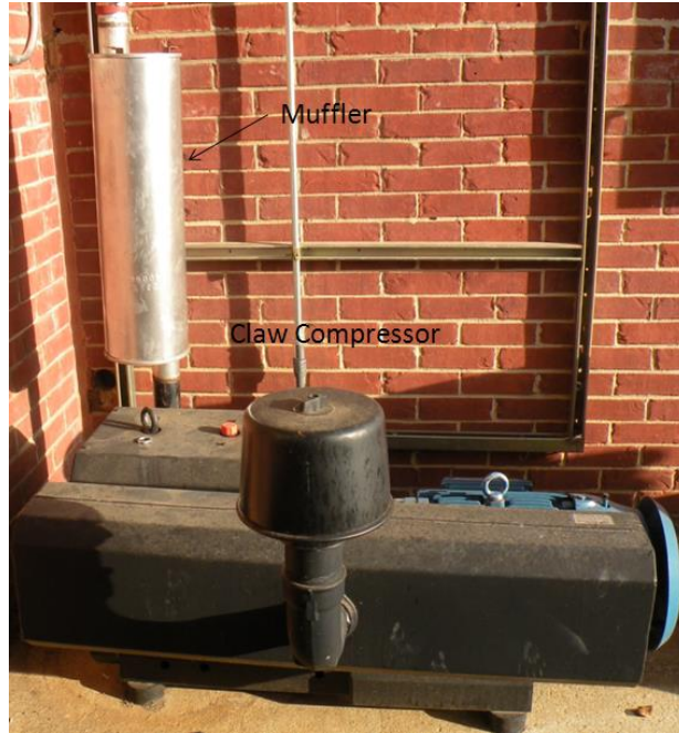
Figure 21 FI test stand claw compressor and muffler
